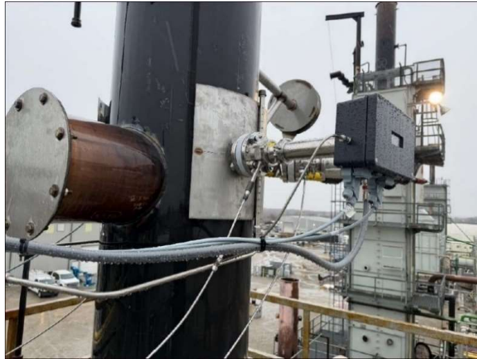
Figure 2 - TDL Analyzer on Test Furnace Stack
