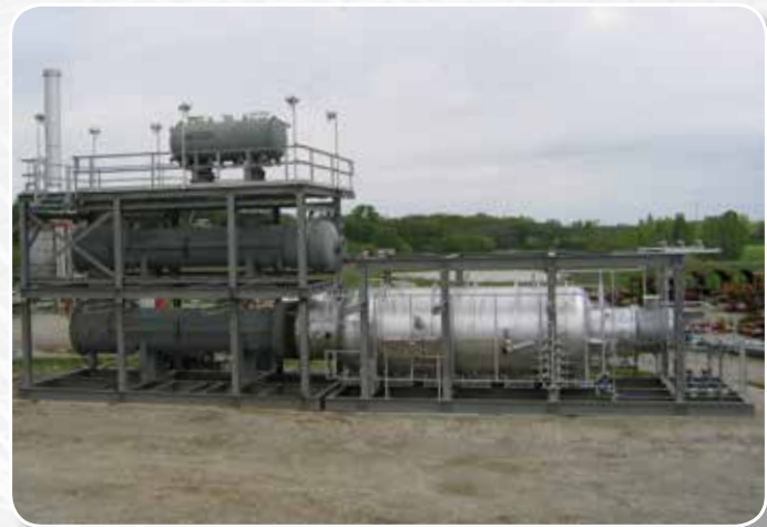
Modularized SRU Reaction Furnace Shipped Pre-Installed on Skid
