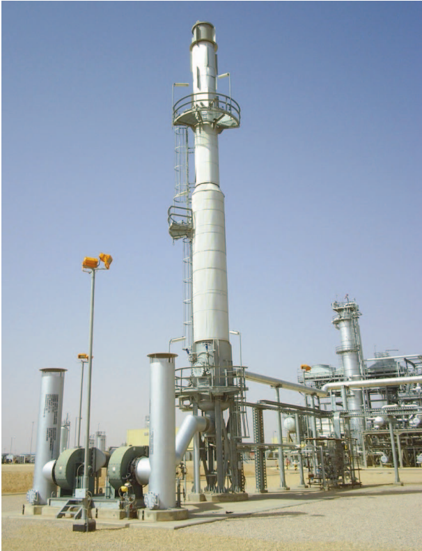
Figure 3. A thermal oxidiser installed at a gas processing plant. Installations such as this one using free jet ultra low NO x burners may achieve NO x levels below 20 ppmv at 3 vol% oxygen.
