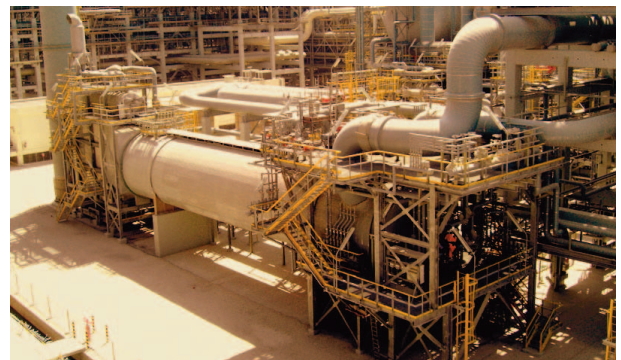
Figure 4. An SRU tail gas thermal oxidiser installed at an LNG processing facility.
